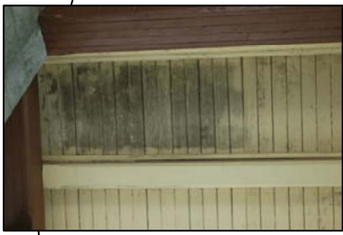
RESTORE DETERIORATING CANOPY CEILING
